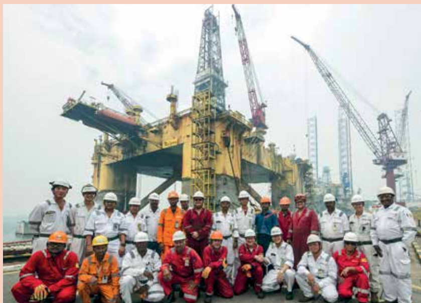
Close cooperation between Keppel and Transocean enabled the repair on Jack Bates to be completed safely and on time
